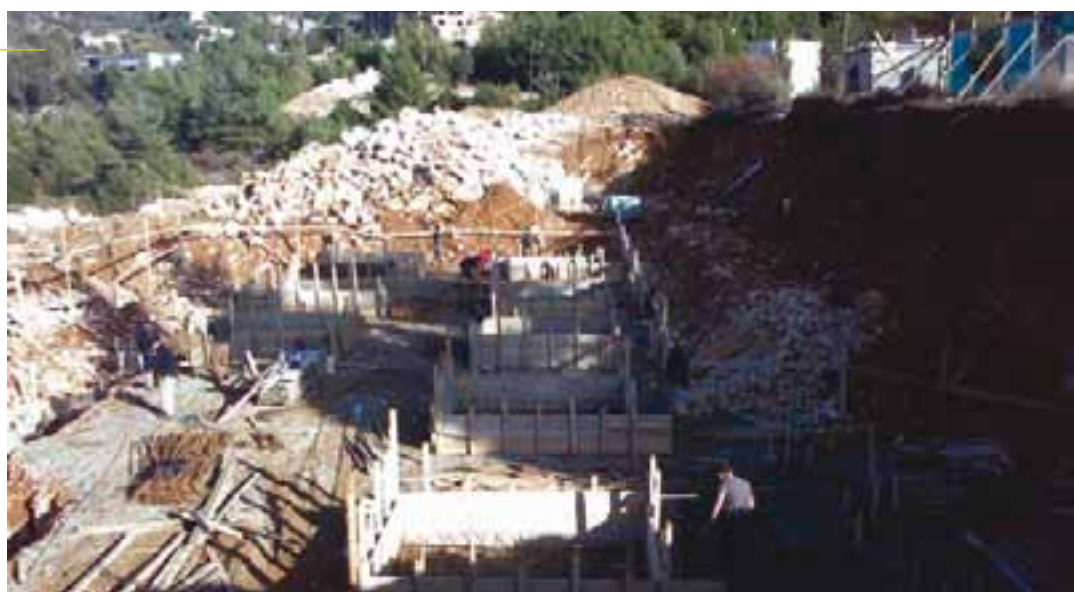
Lebanon, Sebeel Construction of public secondary school of Sebeel - start of the construction
