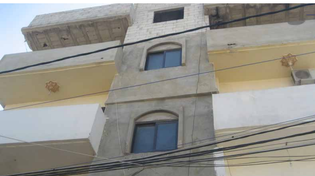
Lebanon, Nahr El Bared. Building under reconstruction. - Housing Repair and Rehabilitation project.
